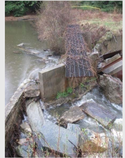
Partially-breached dam on Shoreys Brook
