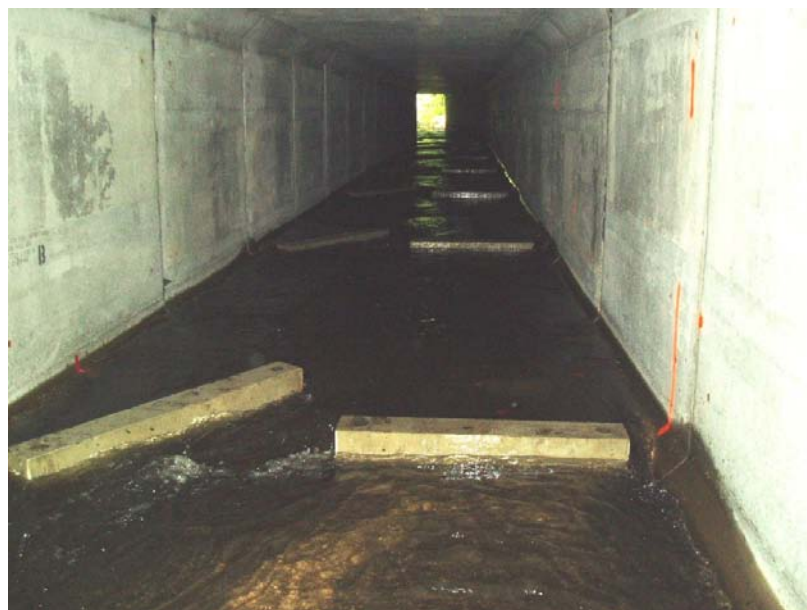
Off-set baffles inside a culvert can reduce velocities and deepen flow to make it passable. In this example, there is a second box with a six-inch lip on the upstream end that diverts all low flow into this box, providing enough water during low flow summer months to pass fish.
